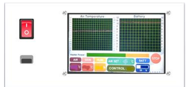
FIGURE 7. Front view of the control panel.
